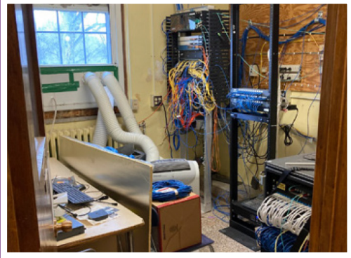
▲ Before: Union Springs MS/HS IDF-4 is a dedicated space that was poorly configured. Floor AC units blocked rack access and cables entered the ceiling unsupported by conduit nor protected by firestop.
